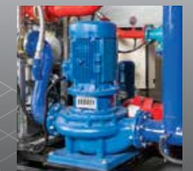
Jacket Water Pump
